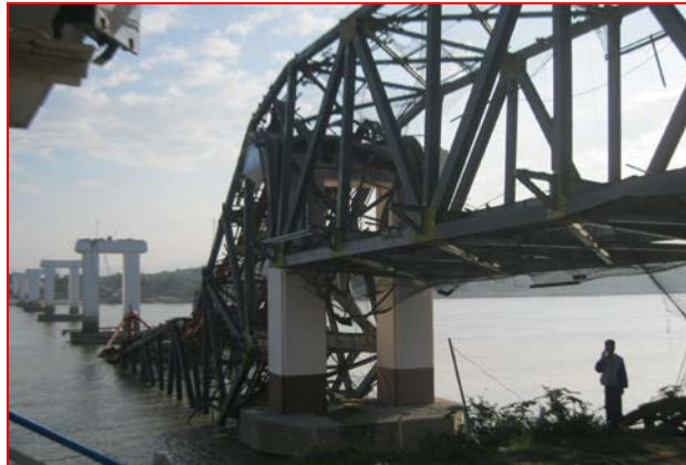
Fig.28. The photo shows a damage of Yardanathingaha Bridge (MEC)
