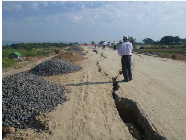
Fig.27. Co-seismic surface deformation: a N-S trending long fissure on the road (Source: MEC)
