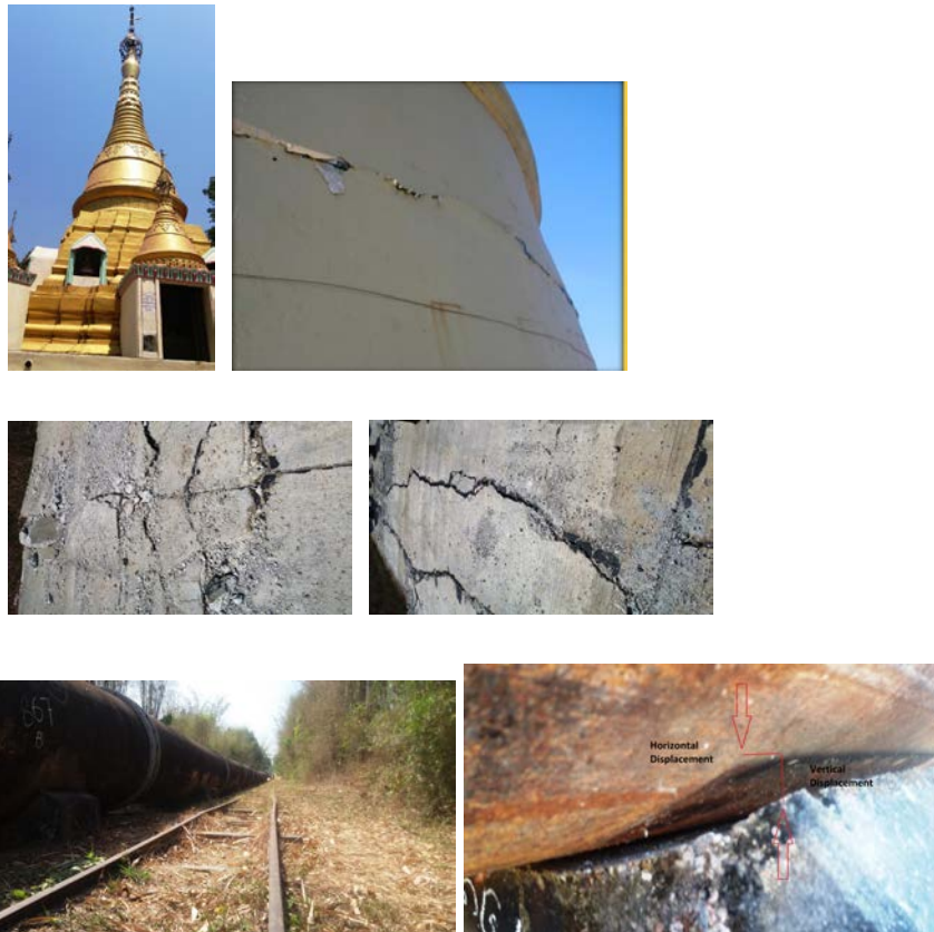
Fig.50 (a). Slight damage to pagoda by the 2017 Taikkyi earthquake (b)Damage to the concrete road and (c) Gyophyu water pipeline by the rupture beneath the surface
