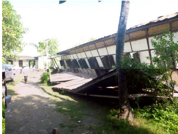
Fig.26. Tilted position of a school is observed during field survey in Thabeikkyin (Source: MEC)
